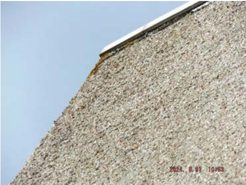
Figure 2.5: Cracking at south elevation
