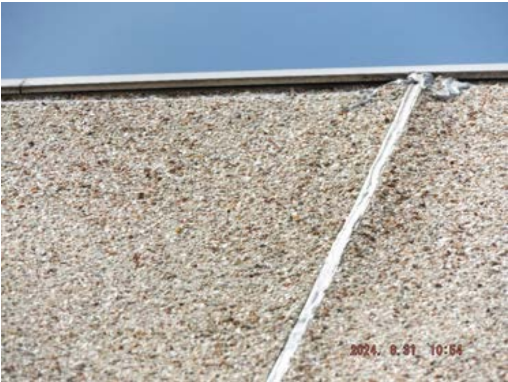
Figure 2.6: Cracking at south elevation
