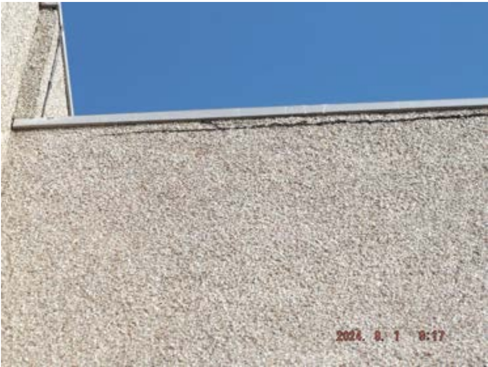
Figure 2.7: Cracking at the east elevation
