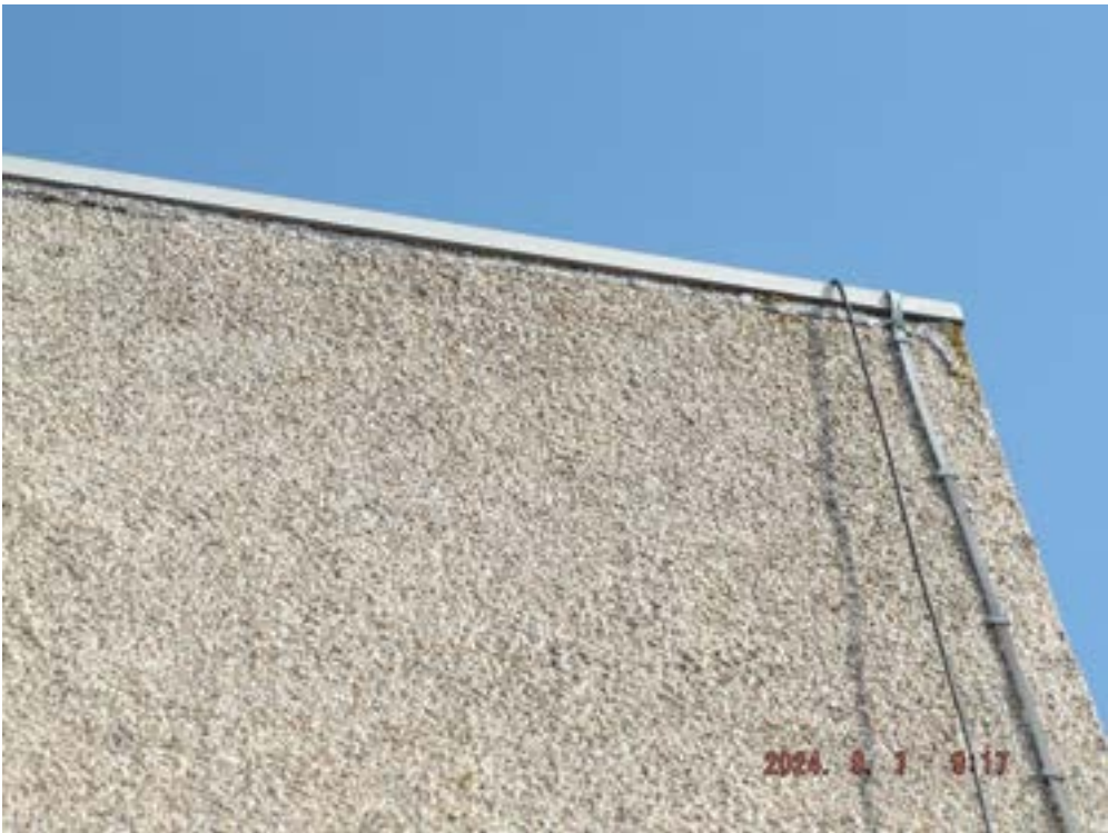
Figure 2.8: Cracking at the east elevation
