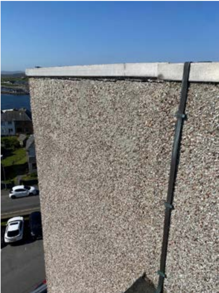
Figure 2.2: Cracking along the east wall head of the lift motor room
