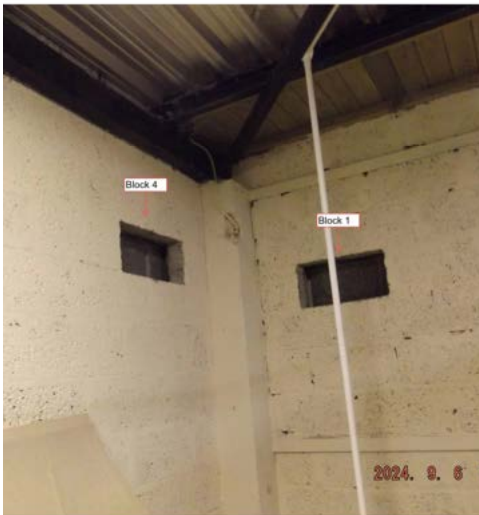
Water Tank Room NE corner
