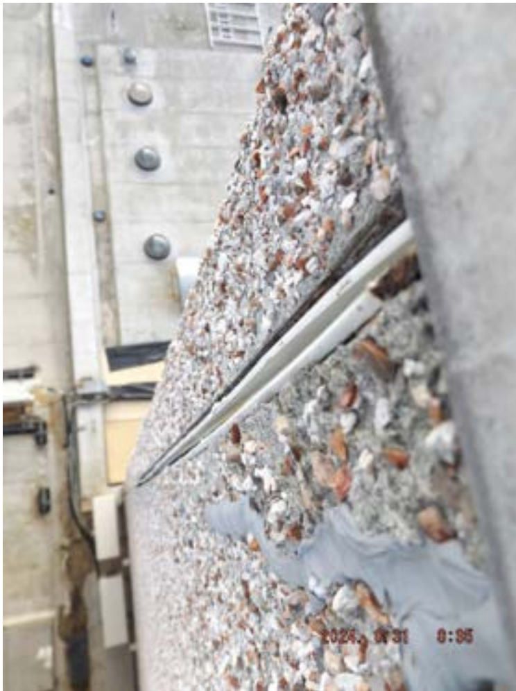
Figure 2.4: Outward lean of the east elevation wall from roof level
